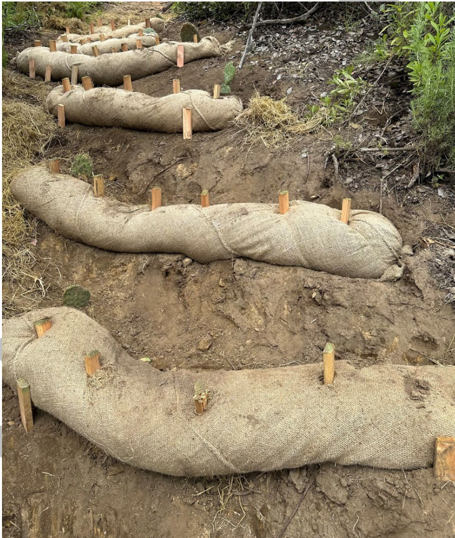
Figure 16: Straw wattles should be densely staked and closely spaced to limit speed buildup.
