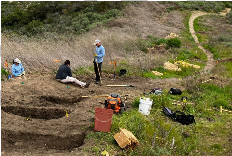
Figure 15: When approached downhill, checkmark ditches should have a gradual entry and an abrupt, nearly vertical exit.
