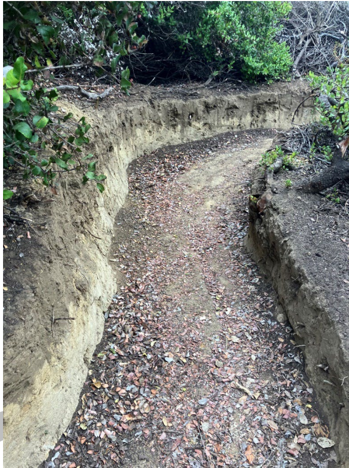
Figure 4: This trench, which reached a depth of 2.5 feet, is an example of destructive trail construction that can permanently damage sensitive cultural and paleontological resources.
