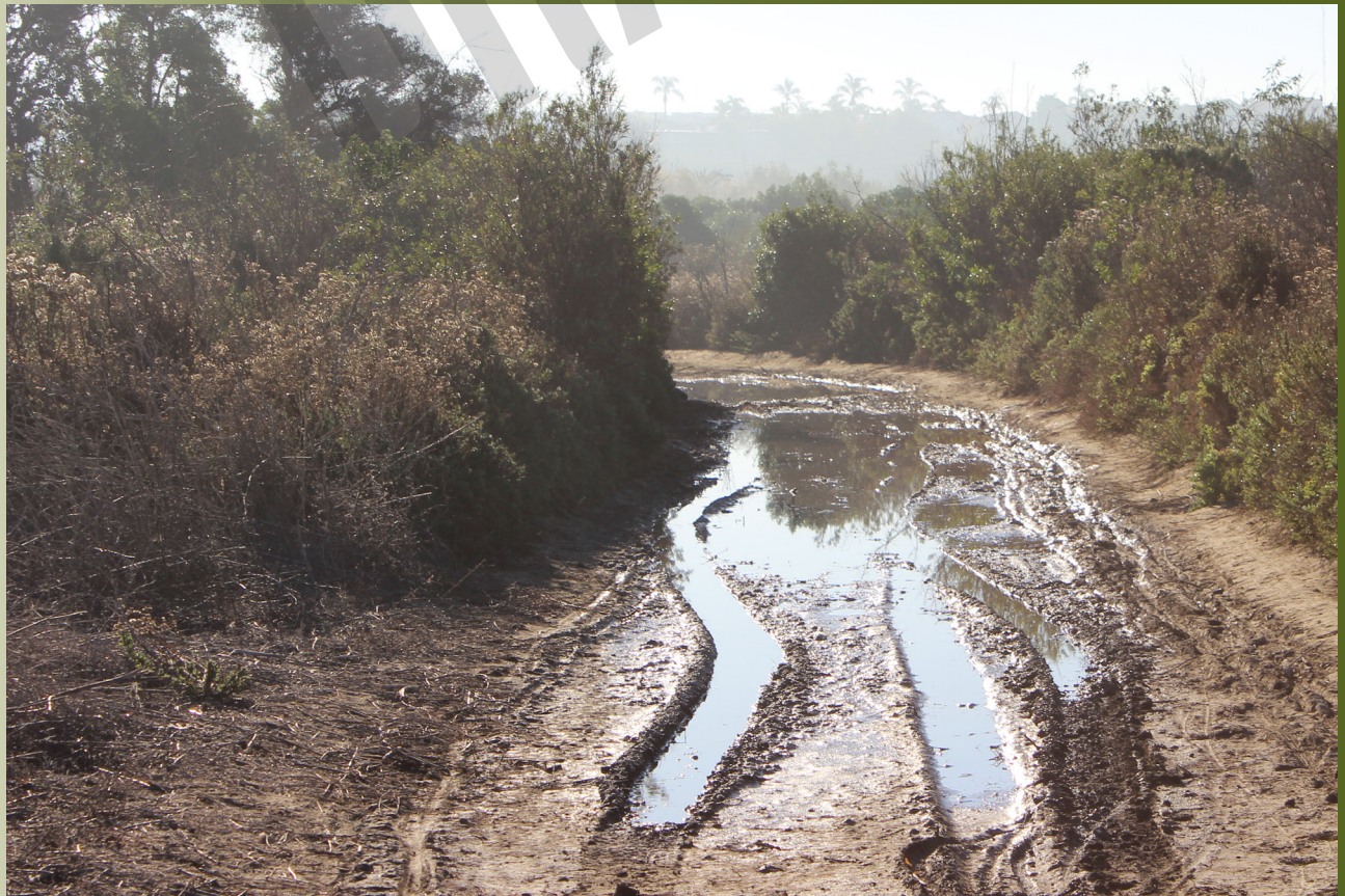
Trail improvements will correct existing conditions causing water to pool in low spots, enhancing emergency responsiveness and pedestrian access.
